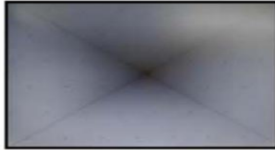
Abnormal Power Section
